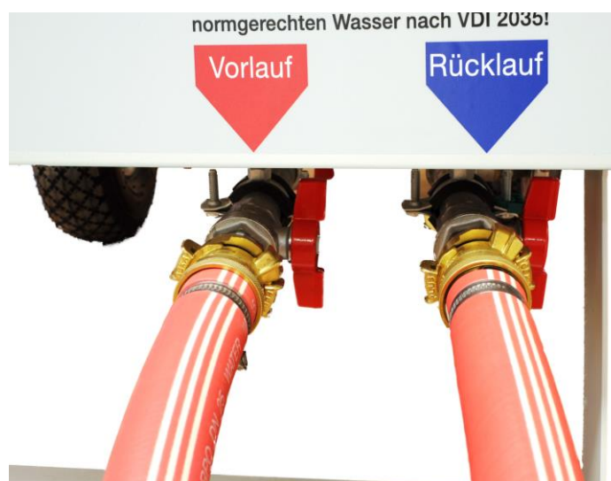
Fig. 8): The DN25 connection hoses on the heating flow (“Vorlauf”) and heating return (“Rücklauf”) of the fittings built into the mobile electric heating unit - fittings are closed -
